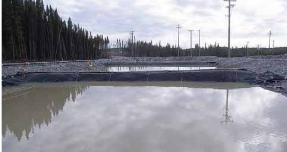
Concrete batch plant settling ponds.
